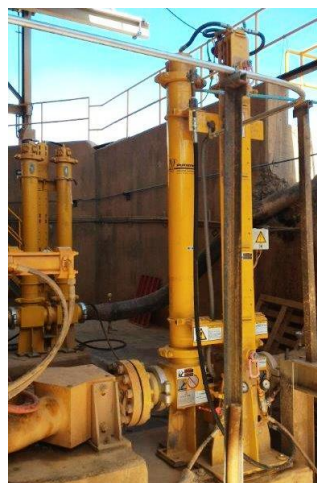
Figure 11: Installed Ventilated Pulsation Dampening System for Tailings Handling
